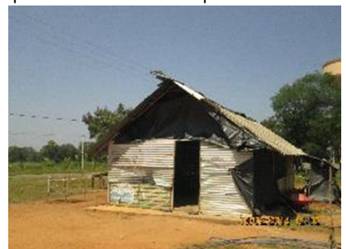
Damaged preschool at Sivanagar
